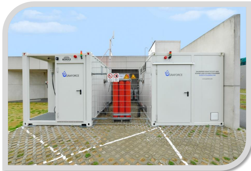
Hydrogen fuel plant from natural gas feedstock
