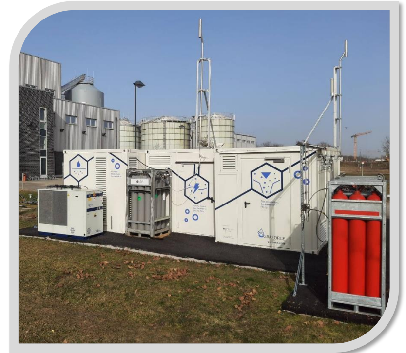
Graforce hydrogen plant from ammonia feedstock
